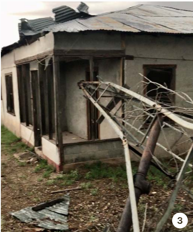
Image 3 caption: Abandoned, dilapidated ranch house with collapsed well support structure and pipe.
