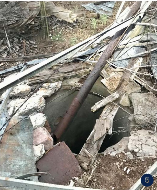
Image 5 caption: Uncovered dry well with broken pipe that once attached to a nearby windmill.
